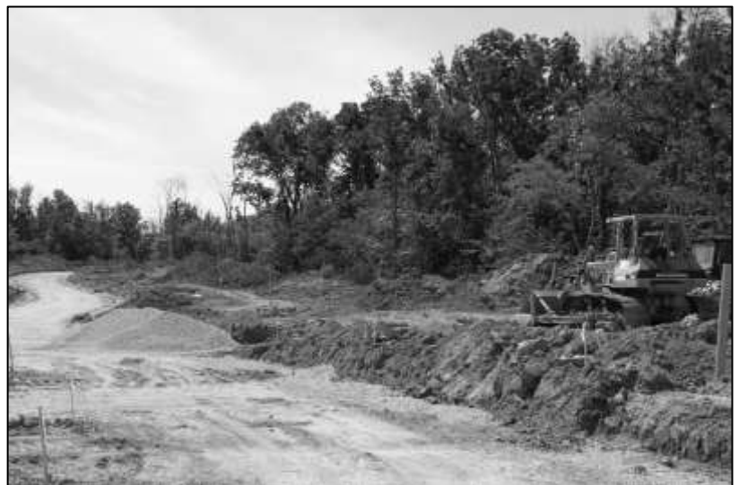
Figure 9: Soil Damaged by Construction
