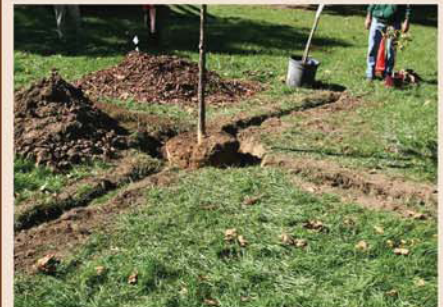
Figure 11 - Larger, established trees can benefit from “radial trenching,” where an Air-Spade or a Supersonic Air Knife is used to dig trenches away from the trunk of the tree in a radial pattern.
